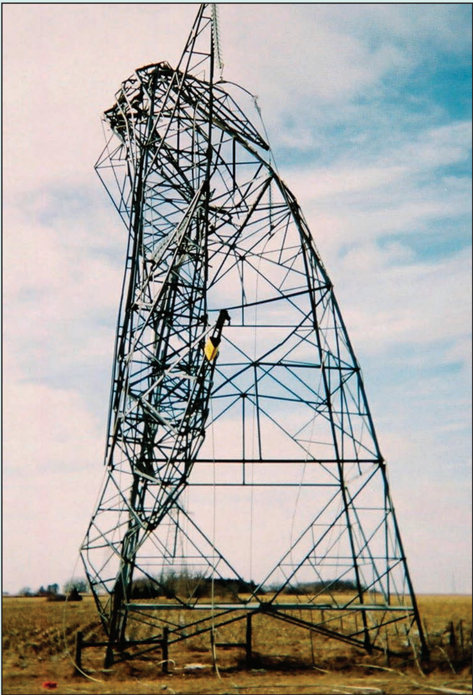
Photo by Jason Gill A collapsed power tower, south of Kearney, after the ice storm through Central Nebraska.
